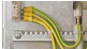
All equipotential bonding conductors are led brought together in the central earthing block.
