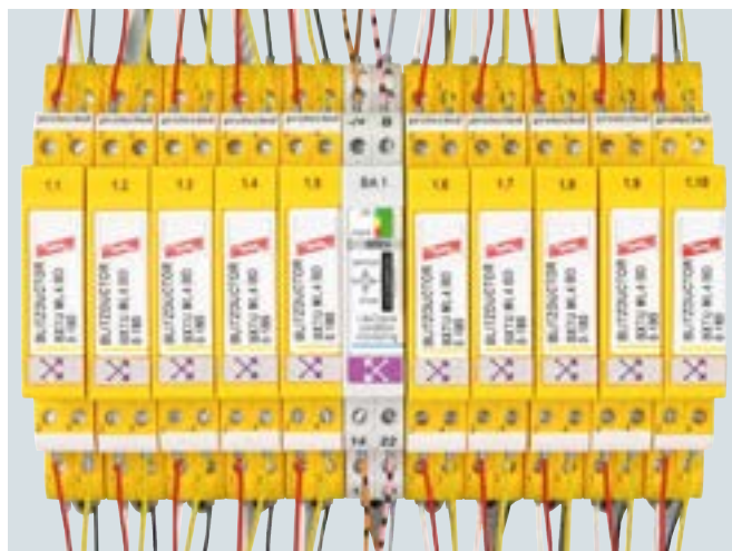
Installed DEHNrecord condition monitoring system
